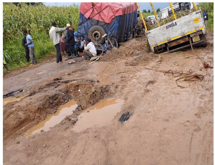
▲ Extensive damage to roads and bridges in Mulanje
