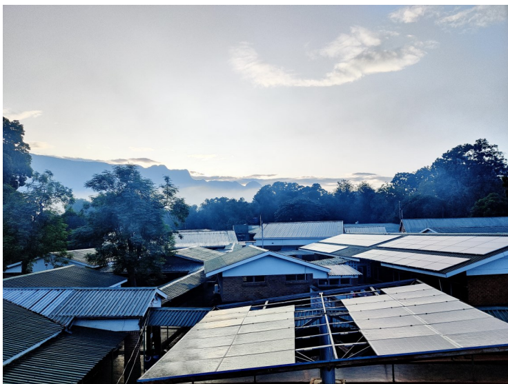
▲ Renovation of the solar trees with in the background new panels in place on OPD
